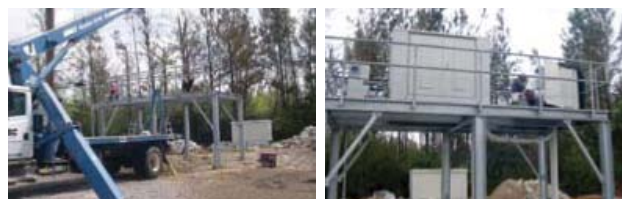
The Tellabs® 1150 Multiservice Access Platform was installed on newly built pedestals on stilts.
